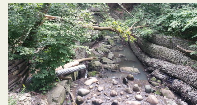
A section of Yellow Creek showing the state of disrepair (c/o scenesto.wordpress.com)
