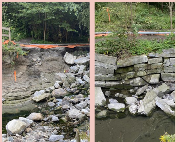
Channel erosion is extensive along Yellow Creek (2 photos below)
